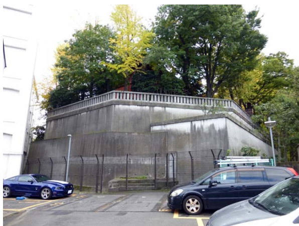
Figure 9: Matsuchi-yama Shoden (Asakusa). The concrete retaining wall that covers the mound behind the temple is shown.
